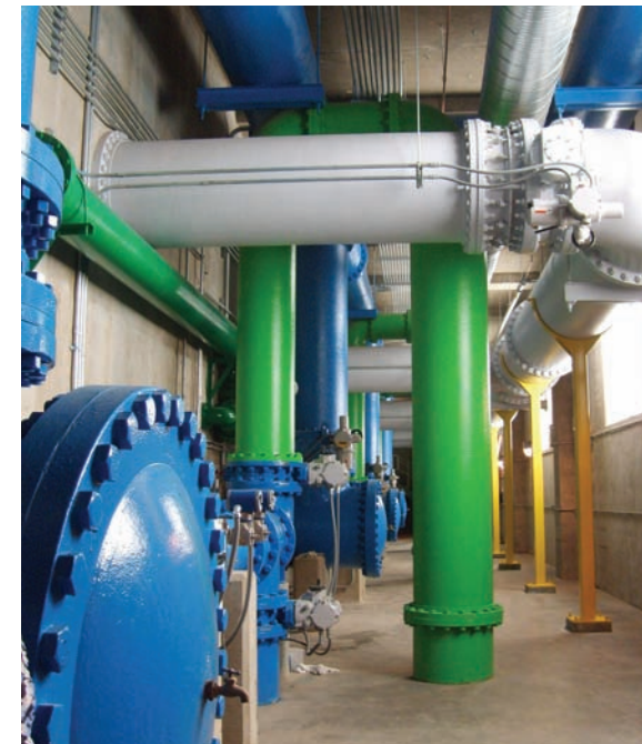
The pipe gallery at the Illinois American Water Champaign water treatment facility.
